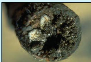
Zebra mussels blocking a pipe
